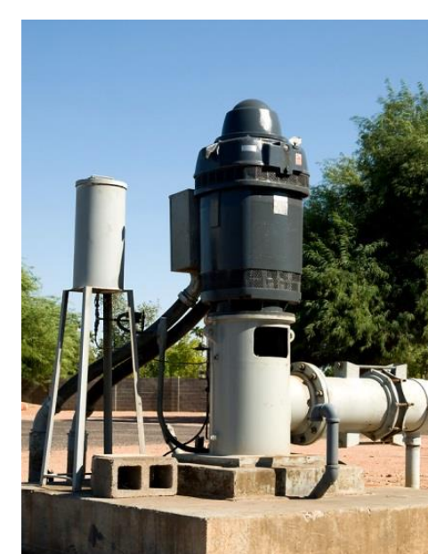
Fig. 2 Town of Gilbert ground water well
