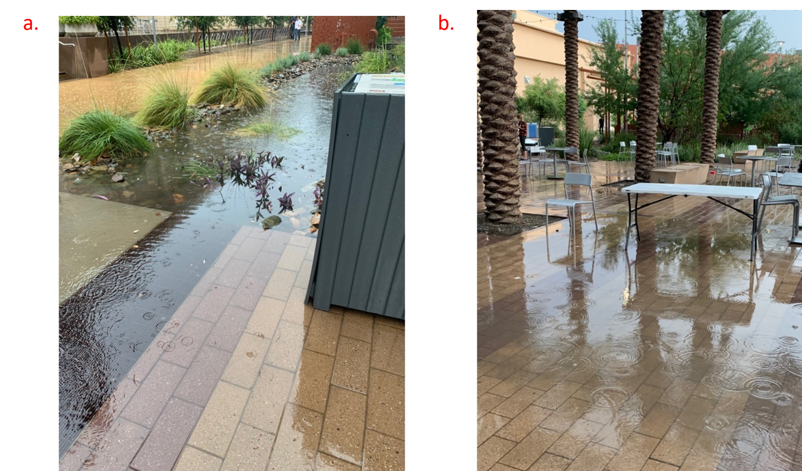
Fig. 6. a) Overflowing basin after heavy precipitation events from July 24-26, 2021. b) Example of water accumulating on impervious surfaces in Orange Mall.
