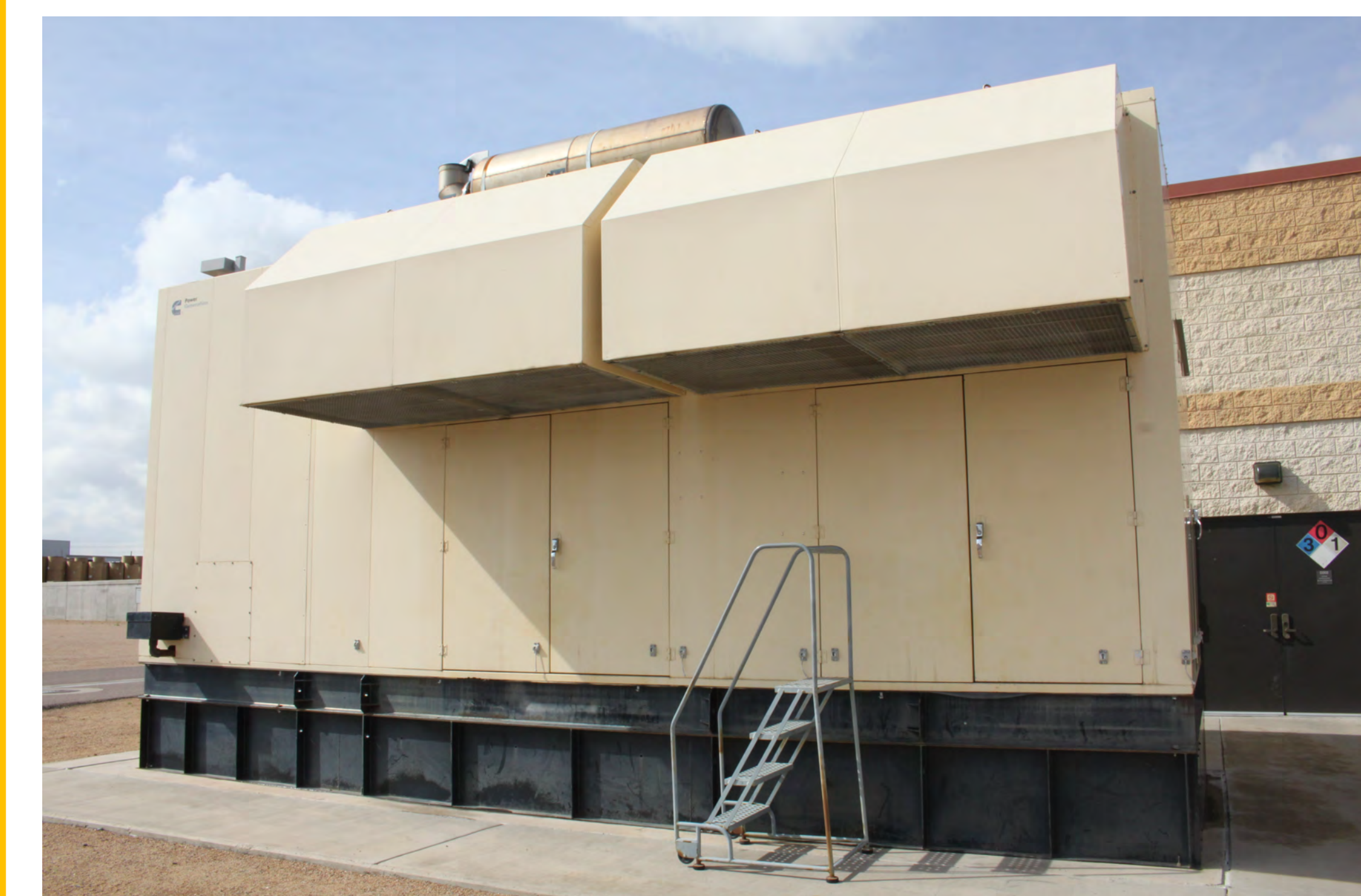
Figure 1: Fuel tank and emergency generator at Glendale Oasis Water Treatment Plant
