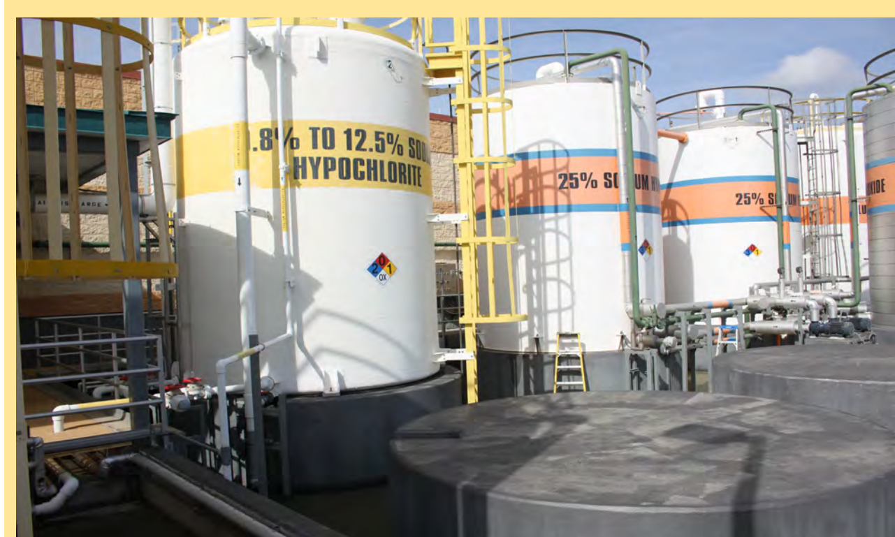
Figure 1: Several ASTs at Glendale Oasis Water Treatment Plant, housed in a secondary containment apparatus
